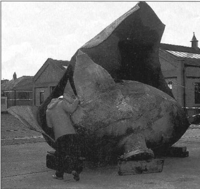
Figure 6-1. The result of an absorber failure. From reference 18. Reprinted with the permission of Gulf Professional Publishing.
